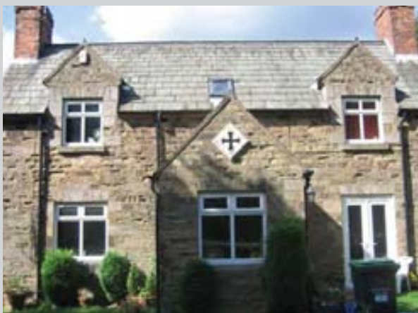
UPVC windows and doors in character properties. This should be discouraged in preference to traditional wooden framed windows and doors.
